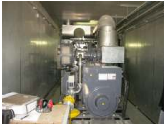
CHP unit within the container
