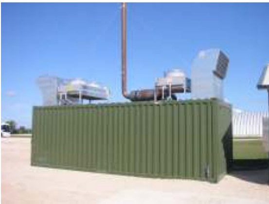
Container housing the CHP unit
